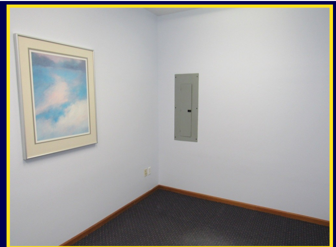
REAR OFFICE WITH ELECTRICAL PANEL
